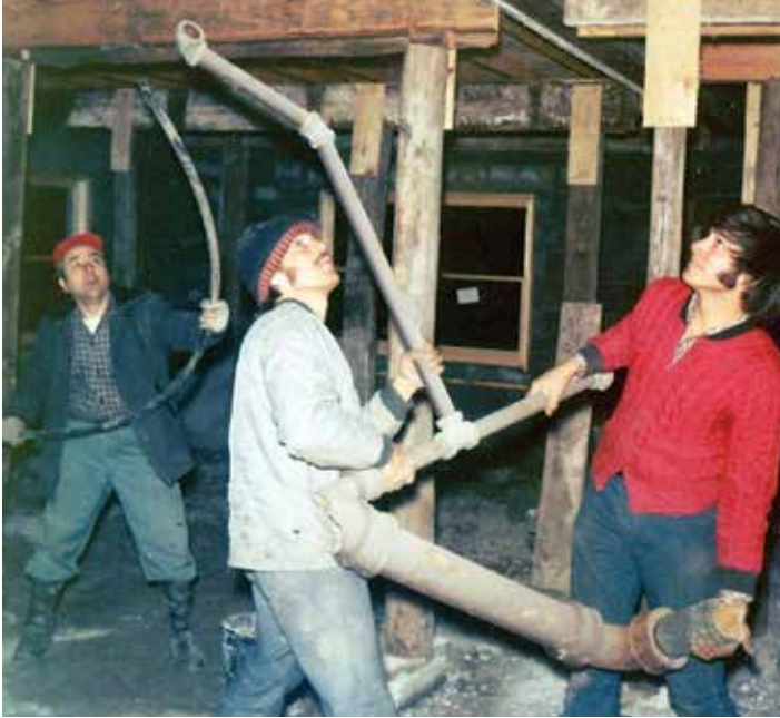
Glenn Zeager, Ken Kurtz, and Les Minninger during the construction of the chapel basement and porch that would later become the Sun Room, 1972.
