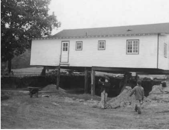
Chapel: second building project at Camp Deerpark was to jack up chapel building and dig a foundation and basement, 1972.
